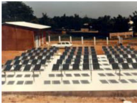
Bifacial solar cell plant in Noto (Senegal), 1988 - Floor painted in white to enhance albedo.
